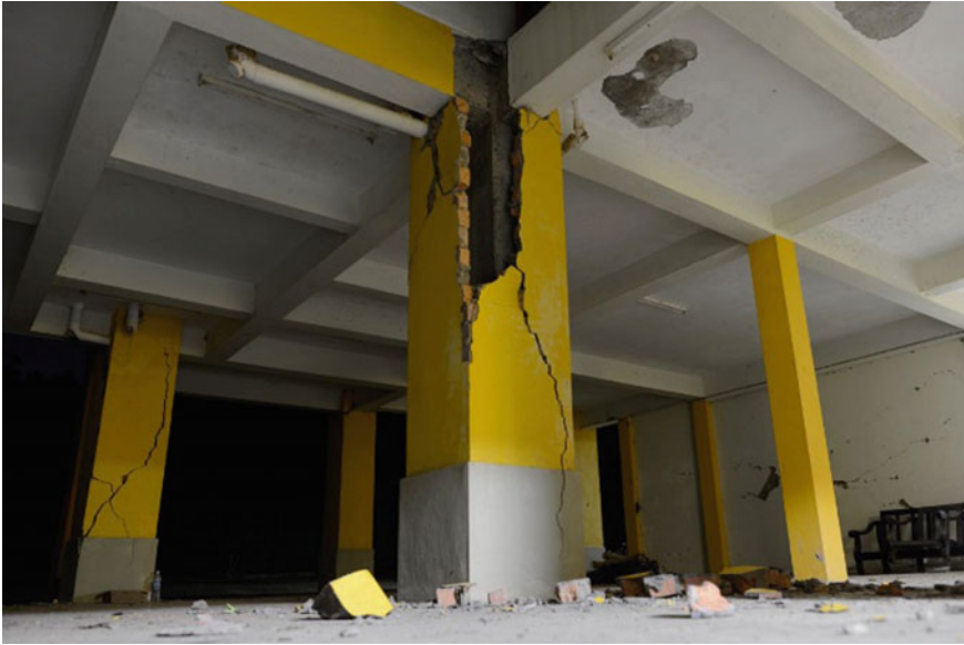
Fig. 1. The damaged column under seismic loading [4]
